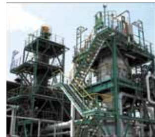
One of the industry's best CFC destruction facilities, which has a capacity of 1,000 tons/year
