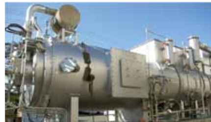
Waste liquid condensation equipment fueled by their own recycled oil (The factory has two units, which are nicknamed "Thomas" and "Percy" based on their appearance.)
