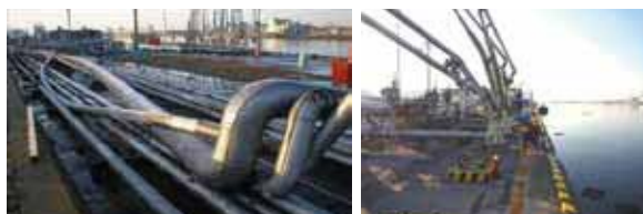
Damage to the berth from the disaster
